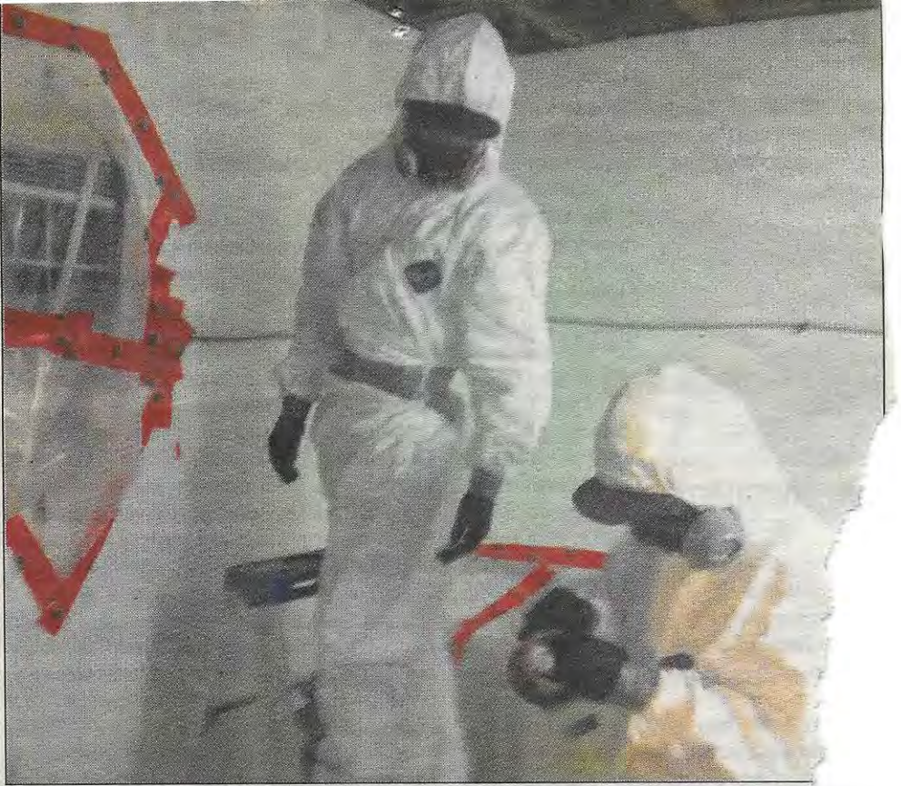
Employees of Jaspro Cleaning Services tackle the removal of mould from the company's head office. The company just became certified in removing asbestos, mould and lead paint.
